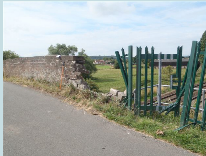
fig2. Infrastructure damage following vehicle collision
